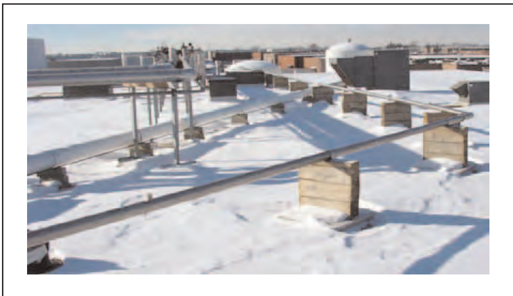
Techniguard vacuum jacketed pipe installed across a plant roof.
